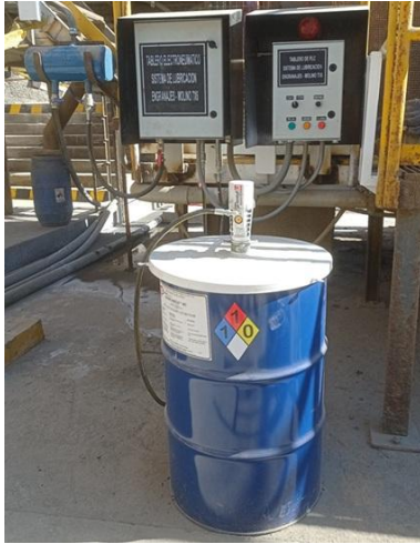
Fig. 2. The electro-pneumatic panel and PLC panel installed next to the drum.
