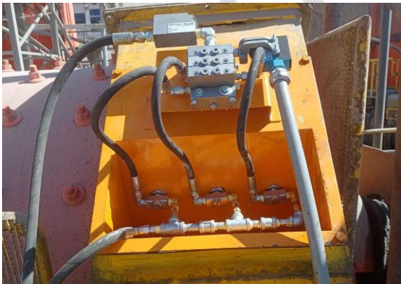
Fig. 3. Valve and sprays panel installed in the gear guard of the mill.
