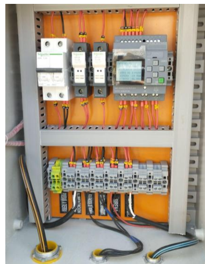
Fig. 5. The PLC panel (inside).
