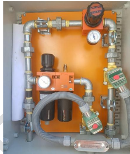
Fig. 4. The electro-pneumatic panel (inside).
